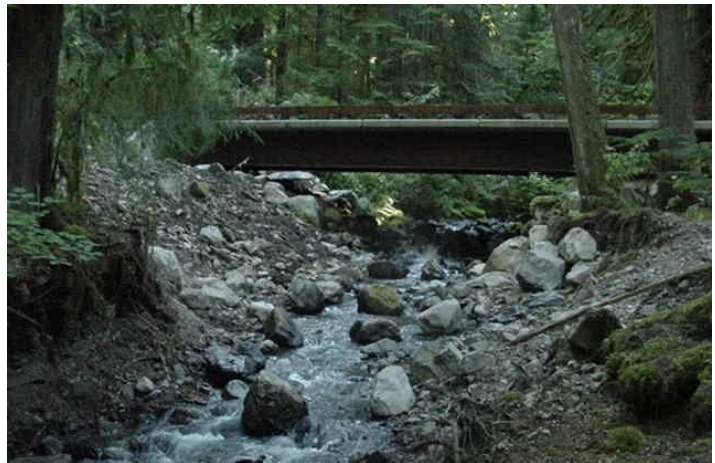
Culvert to bridge upgrade on the Nooksack River. Photo courtesy Mt. Baker-Snoqualmie National Forest.
